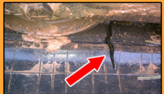
5 Or More Photos Of Failure
